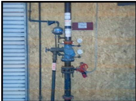
Typical of all three main risers
