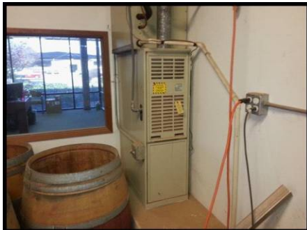
Day & Night gas furnace
