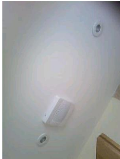
Bathroom-Lighting-Ceiling Mounted Spotlight
