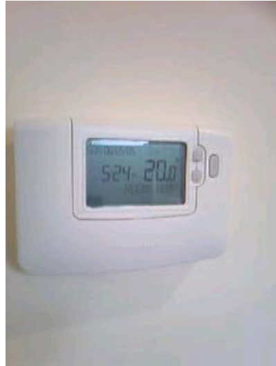
Entrance-Fire and Safety-Thermostat Dial
