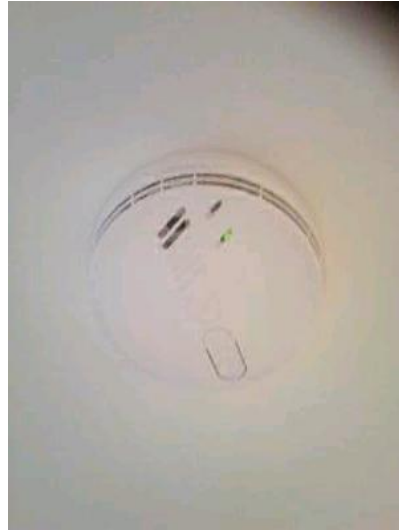
Entrance-Fire and Safety-Smoke Detector
