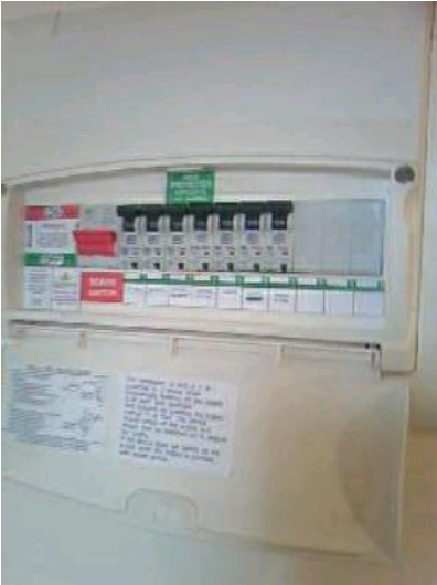
Entrance-Fire and Safety-Fuse Box
