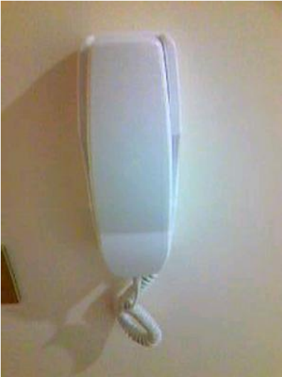
Entrance-Fire and Safety-Voice Intercom
