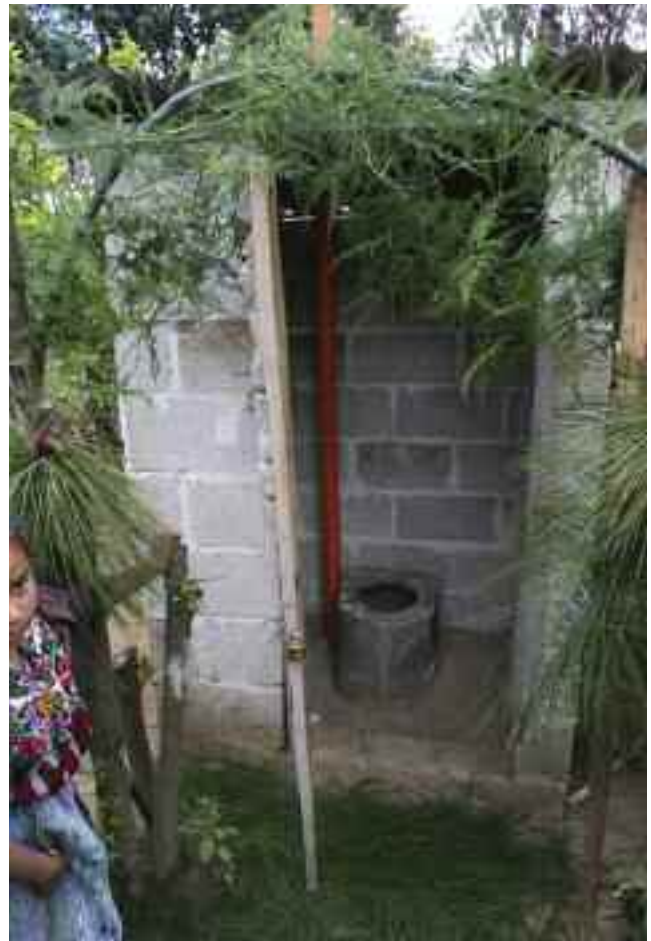
Unsanitary latrines shown in the top photo will be replaced by the vented latrines shown in the photo above. The new latrines are designed to keep flies away and minimize odors.
